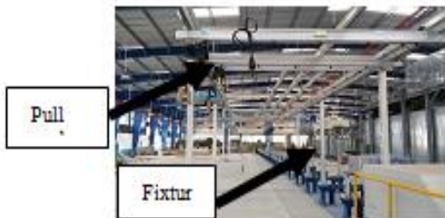
Fig.2. Fixtures on conveyor and pull cord
